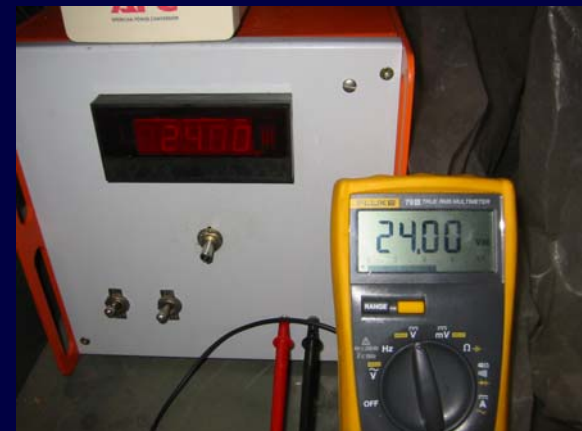
Attach a volt meter to the power supply to verify voltage
